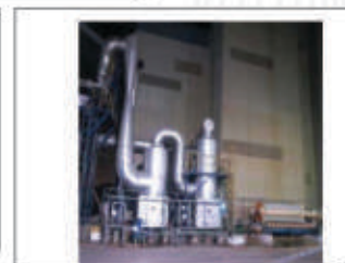
Packed Tower Scrubber
