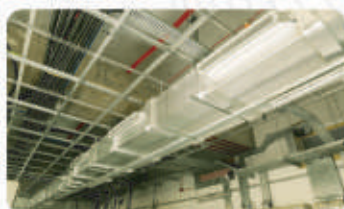
HVAC Duct Insulation
